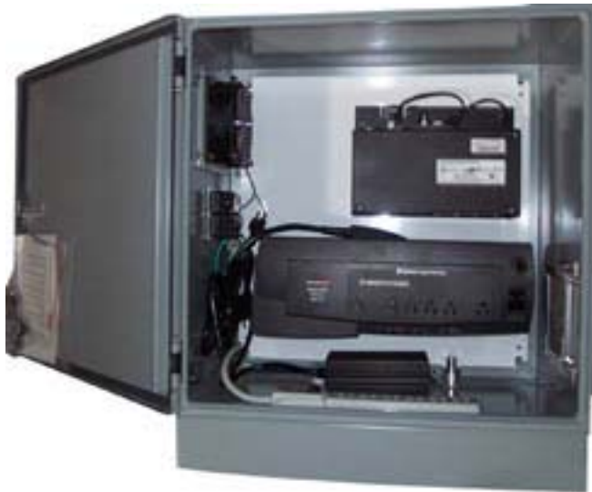
Pic.3 VTC3362 Enclosure with Power UPS and AP
