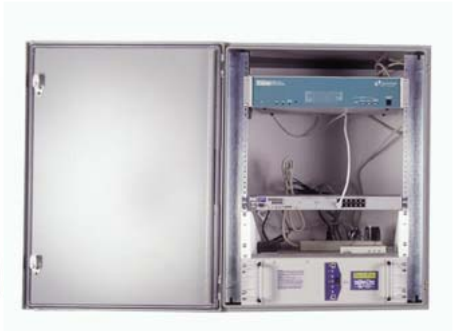
Pic.2. VTC3355 Enclosure with Power UPS, Switch and Tsunami Bridge.
